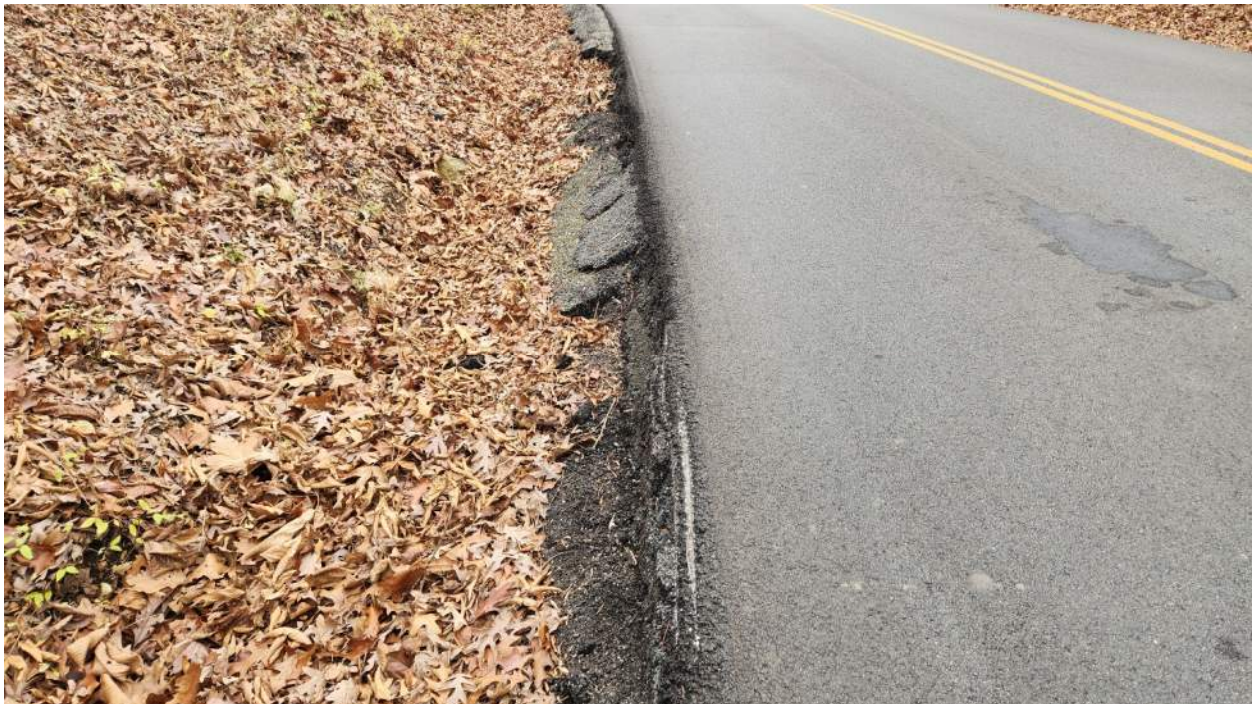
Figure 29 - Pavement edge drop-off east of Patriotic Trail
