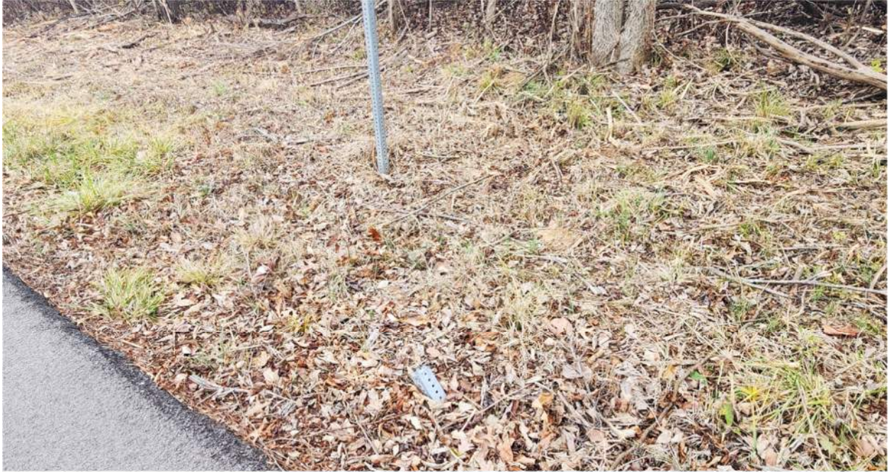
Figure 25 - Broken sign post foundation.
