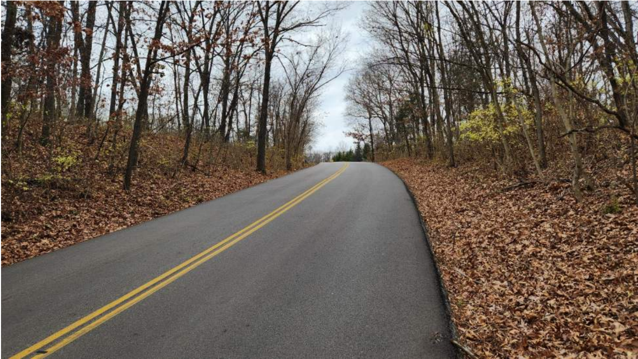
Figure 20 - View looking east back uphill at the curve.
